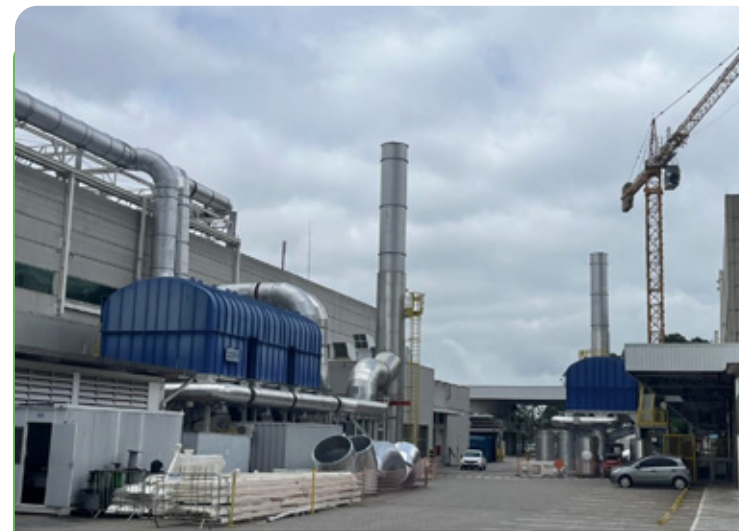
The RTO installation in our Itupeva plant, Brazil
